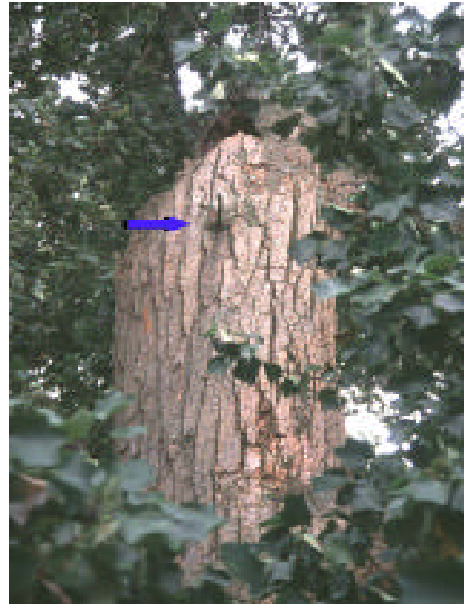
Figure 5: Sixty feet high in the main trunk is an old pruning wound, 32 inches across. The end of a steel bolt protrudes from the side of the limb (blue arrow)
